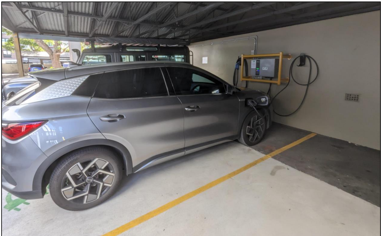
DC Fast Charger – Visitor Parking
